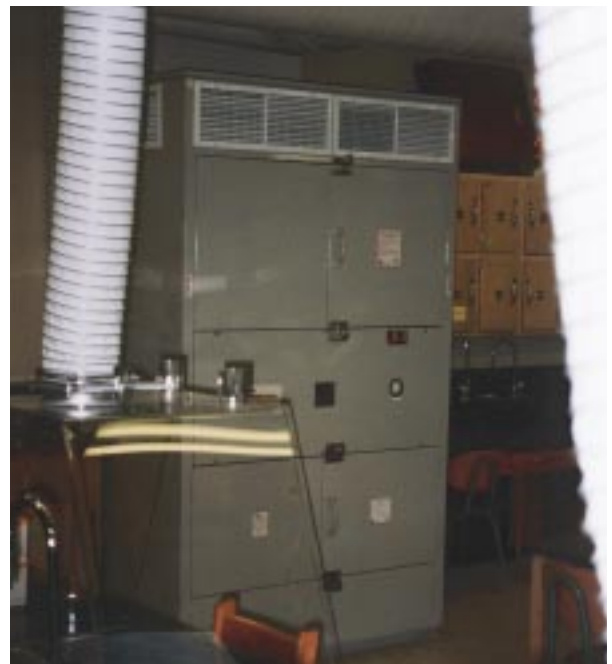
Source Capture Hood System attached to A.P.S.-3000
