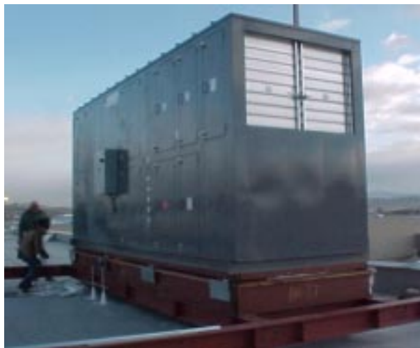
Circul-Aire TMP-15000 unit on airport roof
