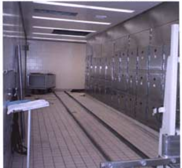
A.P.S.-1500 prior to installation in Main Body Storage area
