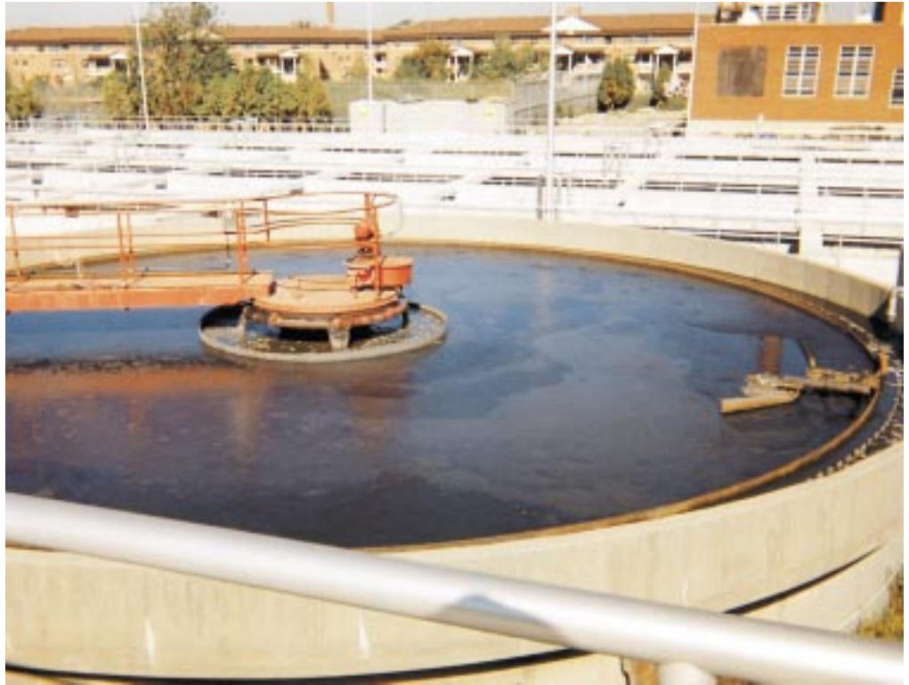
Waste Water Sludge Settling Tank
