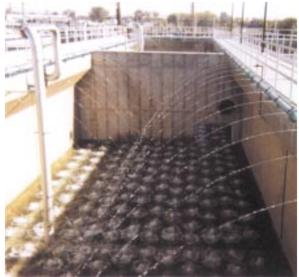
Sewage Treatment Aeration Process
